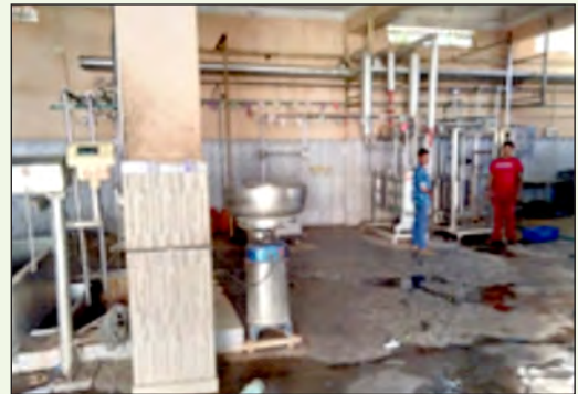
Milk Processing Plant
